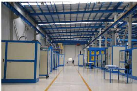
年产10000套应力锥的世界一流注橡系统 Over 10000 accessories each year from this equipment
